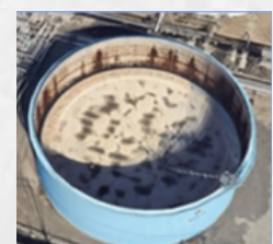
External Floating Roof
